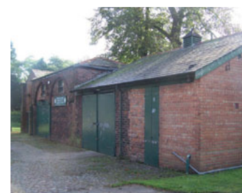
'Coach House' fully restored. To be a multi-functional building; see Board D for more details
