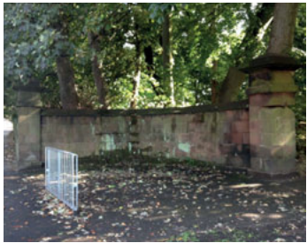
Entrance feature; eastern side, c. 1760 feature : Repair + reinstall the missing pillars + wall
