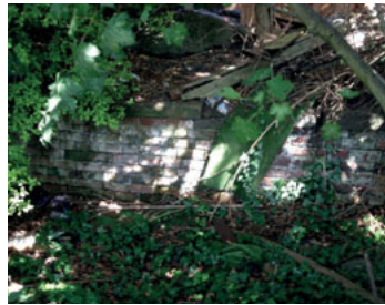
Ha-ha : c. 1760 feature : Repair wall + coping, remove hedge on top + reinstate the ditch
